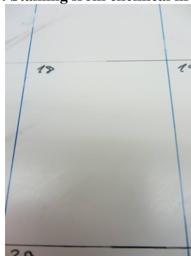
18: Staining from chemical nr. 17
